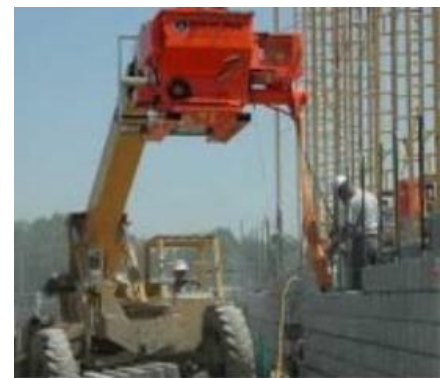
Grout delivery system
