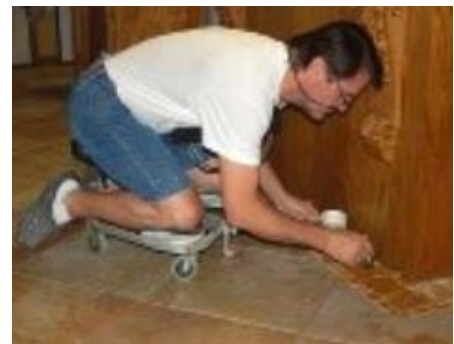
Performing detail work at floor level while positioned on a knee creeper
